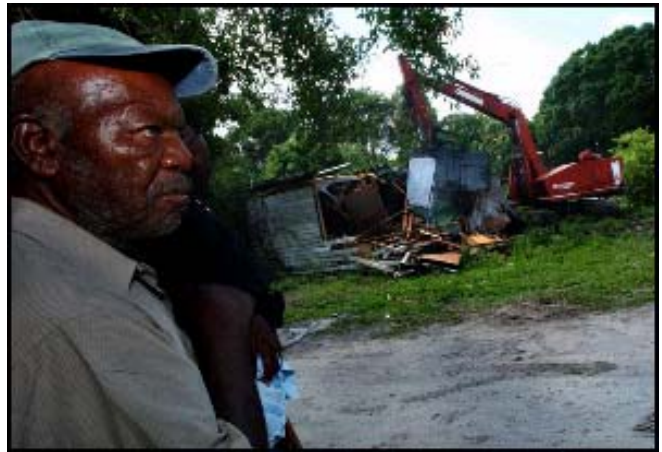
Wiggs watches as workers from Affordable Trucking & Land Clearing Inc. of Wabasso demolish his house Tuesday. Wiggs will be getting a new house built for him as part of an effort to improve the living conditions in the area through a multi-agency project.
